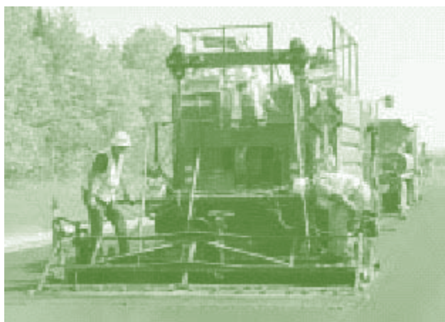
Microsurfacing on Interstate 75 in Michigan—one of 14 pavement preservation techniques in FHWA's program.
