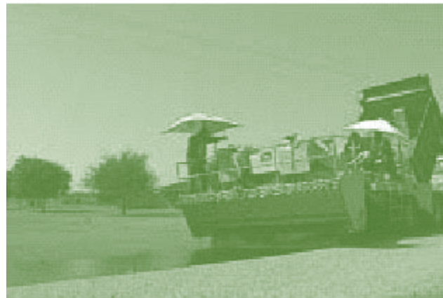
Chip sealing protects new pavements, increases macrotexture, and prolongs the life of structurally sound pavements that show surface distress.
